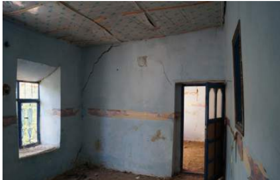
Fig. 2-4. Damages formed on the junctures of internal & external walls
