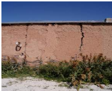
Fig. 2-1. Vertical cracks and opening damages on the external wall
