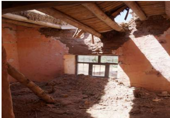
Fig. 2-5. Damages formed on the wall junctures of the beams of the roof
