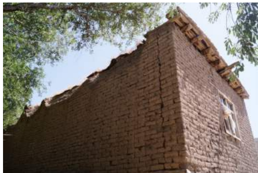
Fig. 2-3. Damages on the corner junctures on the external walls
