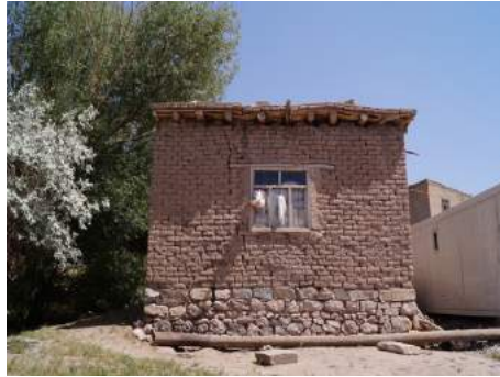
Fig. 2-2. The formation of damages as a result of the window spaces in the external walls
