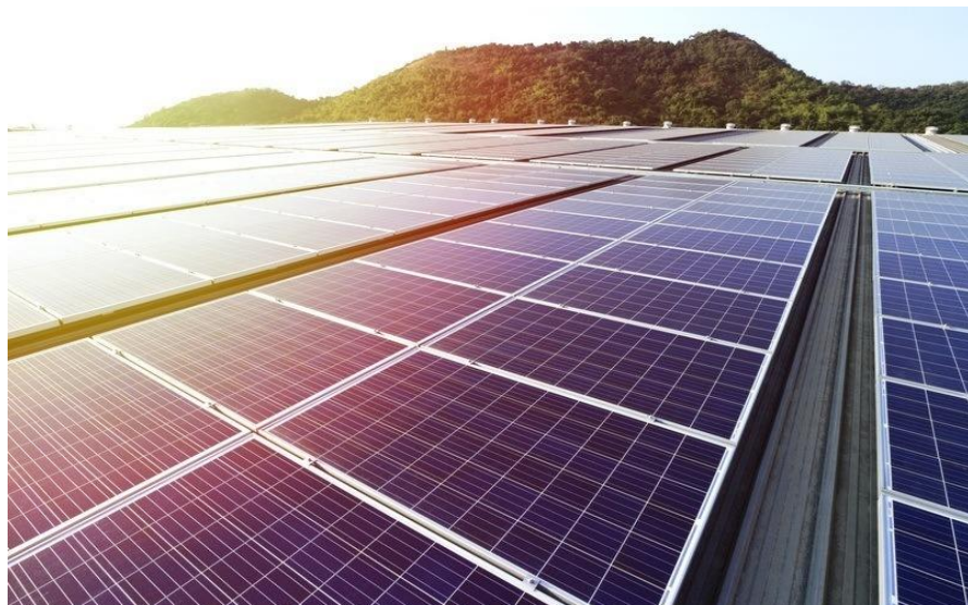
Figure 2 Solar PV system used for electricity generation.
