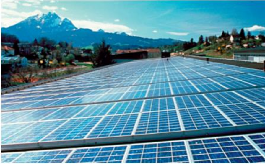
Figure 1.1: A large array of PV modules on a rooftop in Switzerland.
