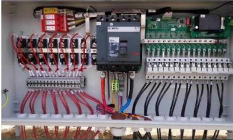
Figure 13: Connecting box at QASP Bahawalpur [61]
